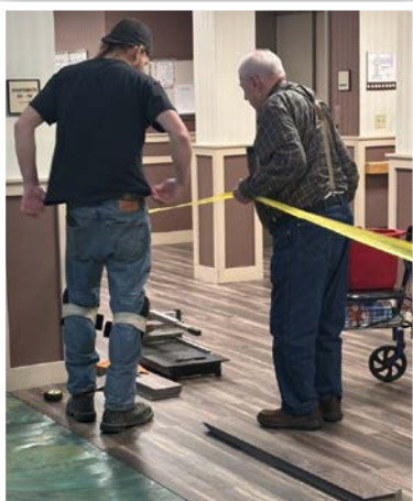
▲ Ron supervising the construction work as they put in new flooring at PAV.
